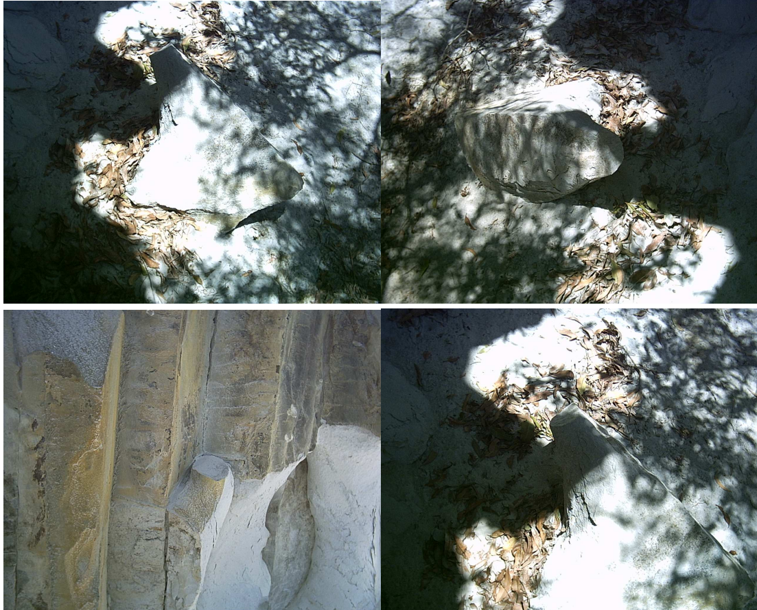
Figure 99. Montage - Fallen Block, East face
