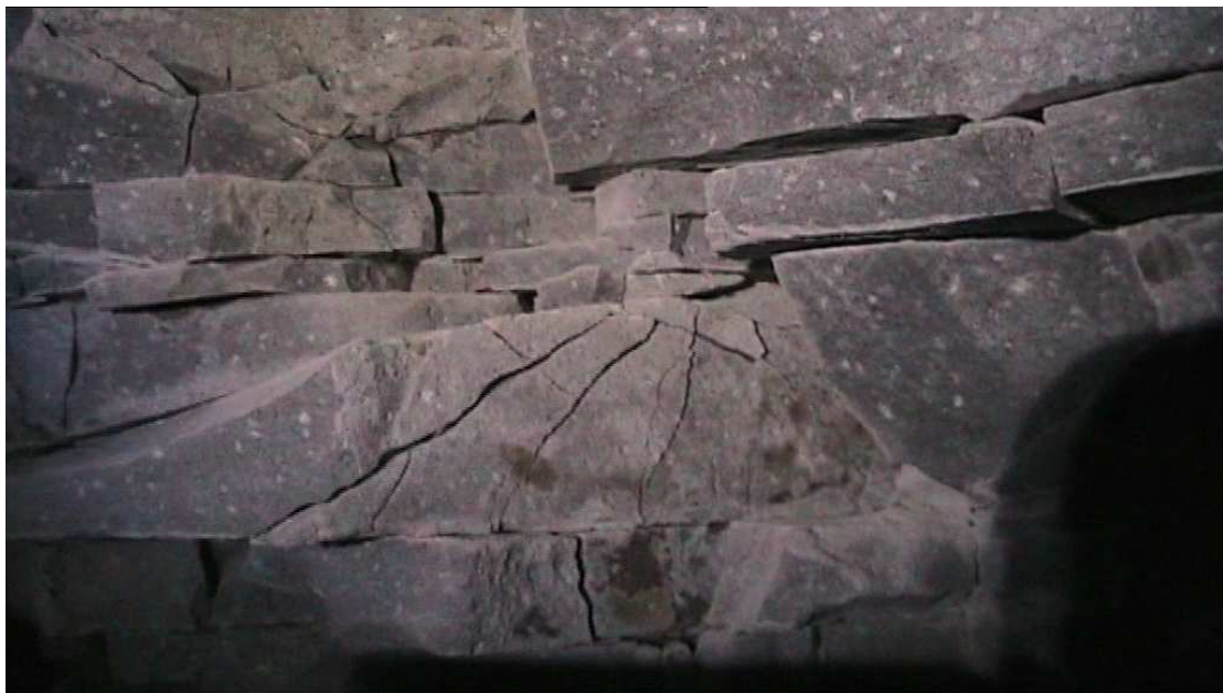
Figure 164 A stress cracking pattern identified to the right of the archway of perched shale plates at the top of the rear of the cave
