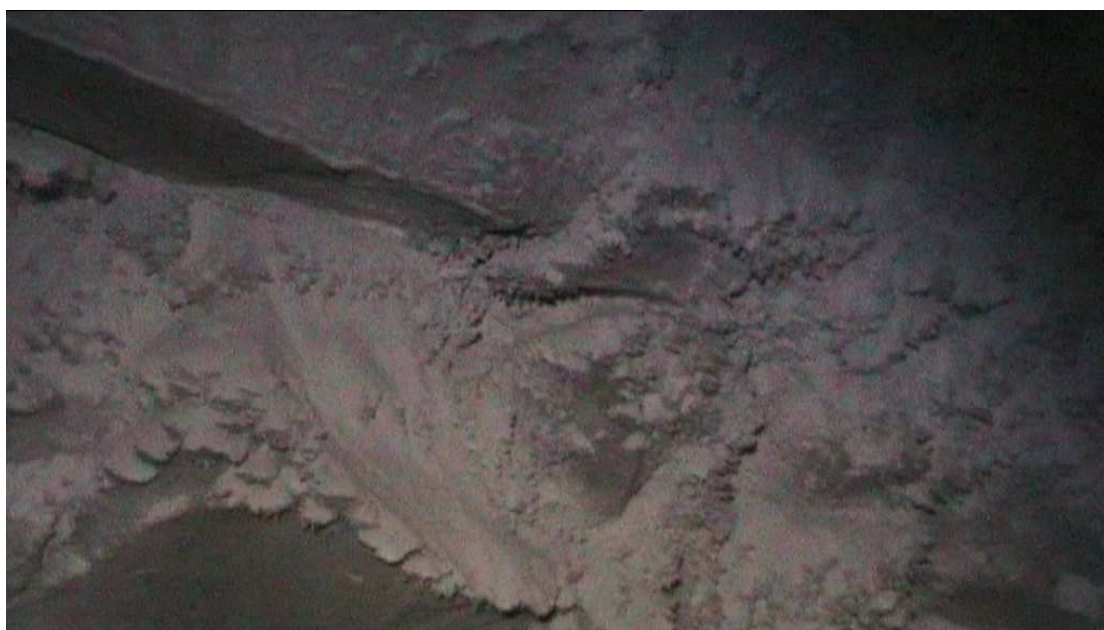
Figure 158. Crumbly brittle rock
