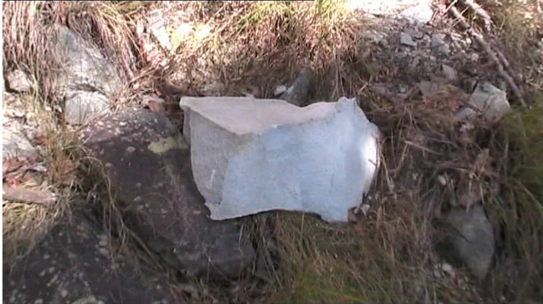
Figure 100. Fallen block, East face
